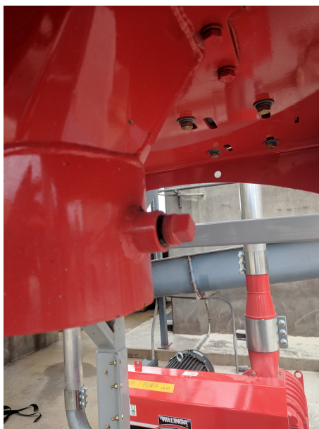
Figure 2: Plugged Sensor Port
