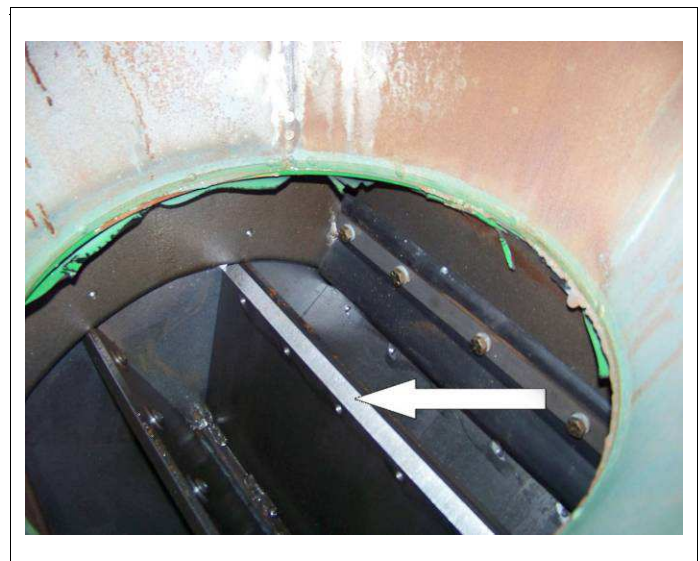
Fig. 5-29 Checking Tip Clearance Through The Access Door.
