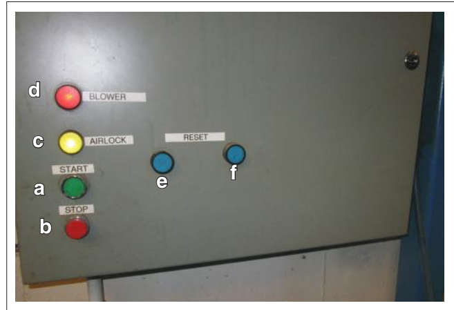
FIG. 2 MASTER CONTROL PANEL
