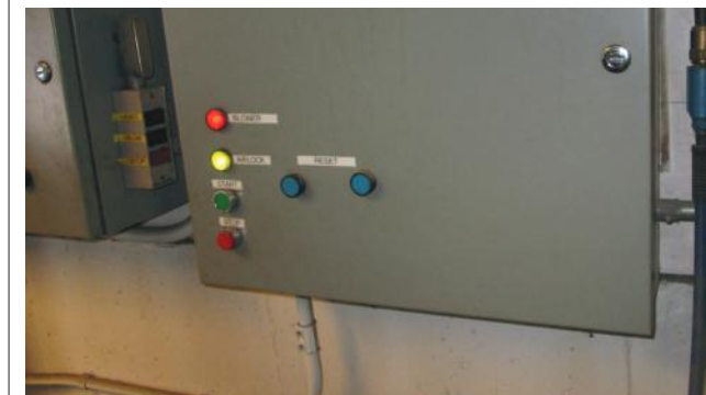
Master Control Panel
